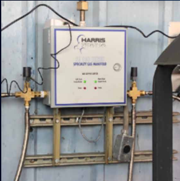
6000psi (410bar) pressure sensor on Nitrogen manifold
