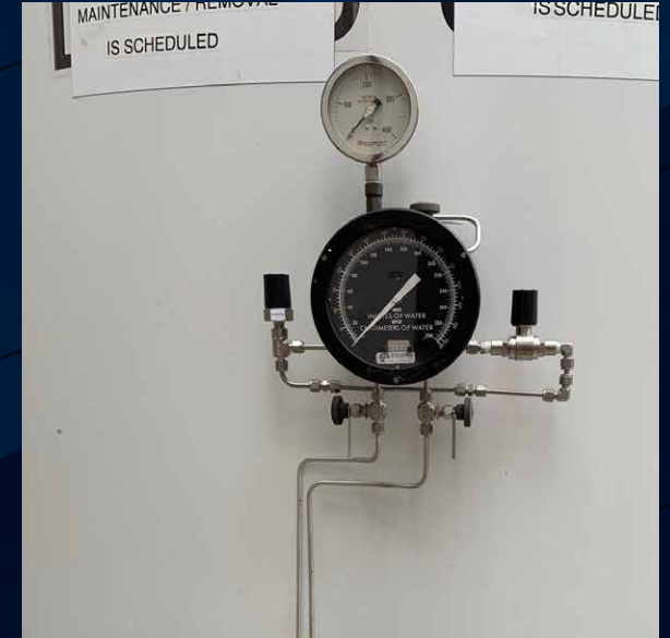
Level + Pressure Sensor on Cryo Tank
