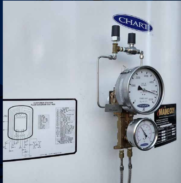
Differential Pressure (Level) Sensor + Pressure Sensor on Cryo Tank
